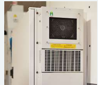
Heat Exchanger for Electrical Cabinet
